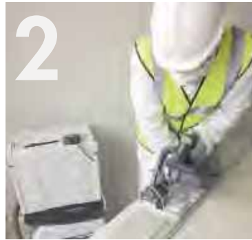
2 Cutting the edge of the first board with a circular saw fitted with a dust extractor.
