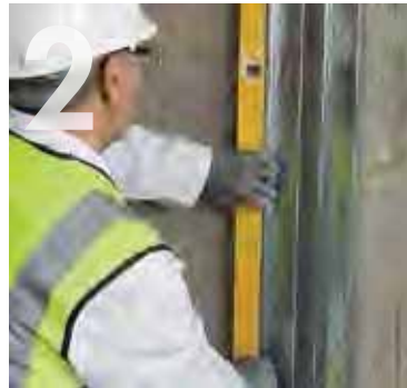
2 After fixing the head track, the floor track should be positioned by using a vertical stud and a spirit level.
