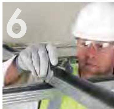
Connecting lower and upper Knauf 'C' Channel with Knauf Channel Intersection Connectors.
