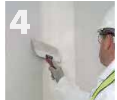
Apply Knauf Joint Cement Easy Sand finish coat to 75mm each side.
