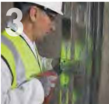
3 Bracing Knauf 'C' Studs with Knauf Fixing Channel at maximum 1500mm vertical centres (if required).
