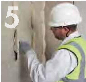
Applying Knauf Plasterboard Adhesive around the perimeter and at the required centres.
