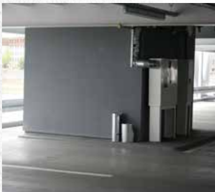
Car Park Utility Rooms | Stuttgart, Germany
