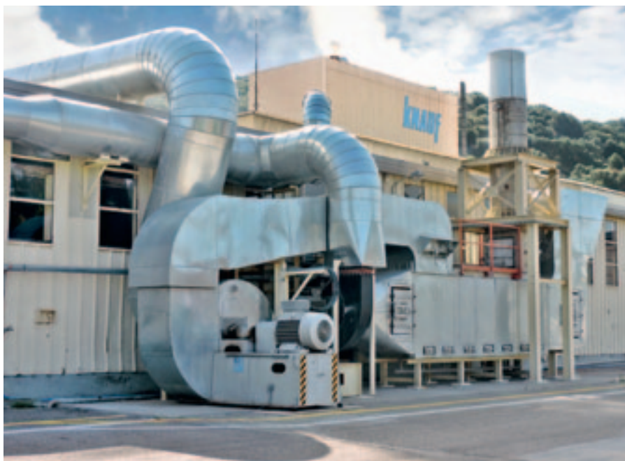
Cogeneration plants help save energy and increase energy efficiency.
